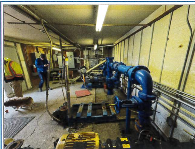
Pump Station Interior
