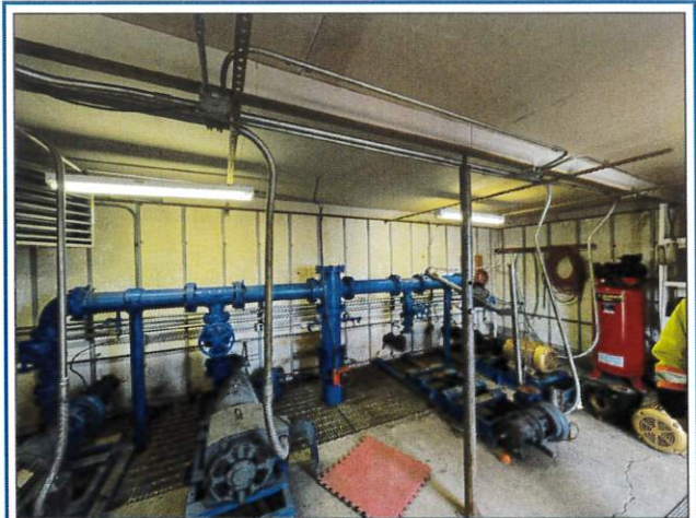
Pump Station Interior
