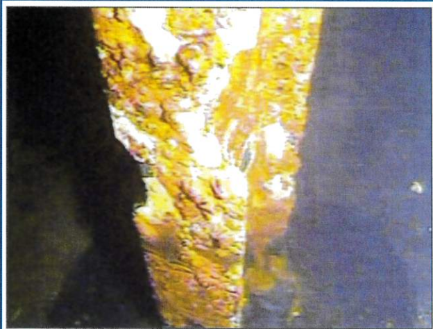
Roof Support Column Submerged
