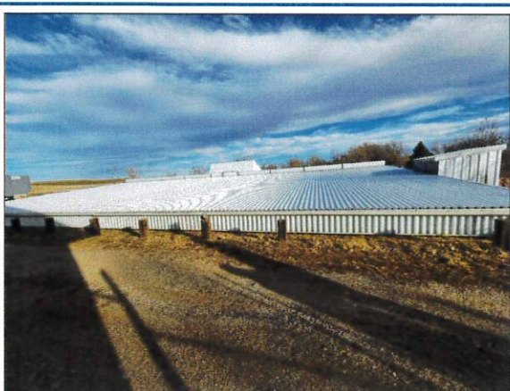
Semi Buried Reservoir
